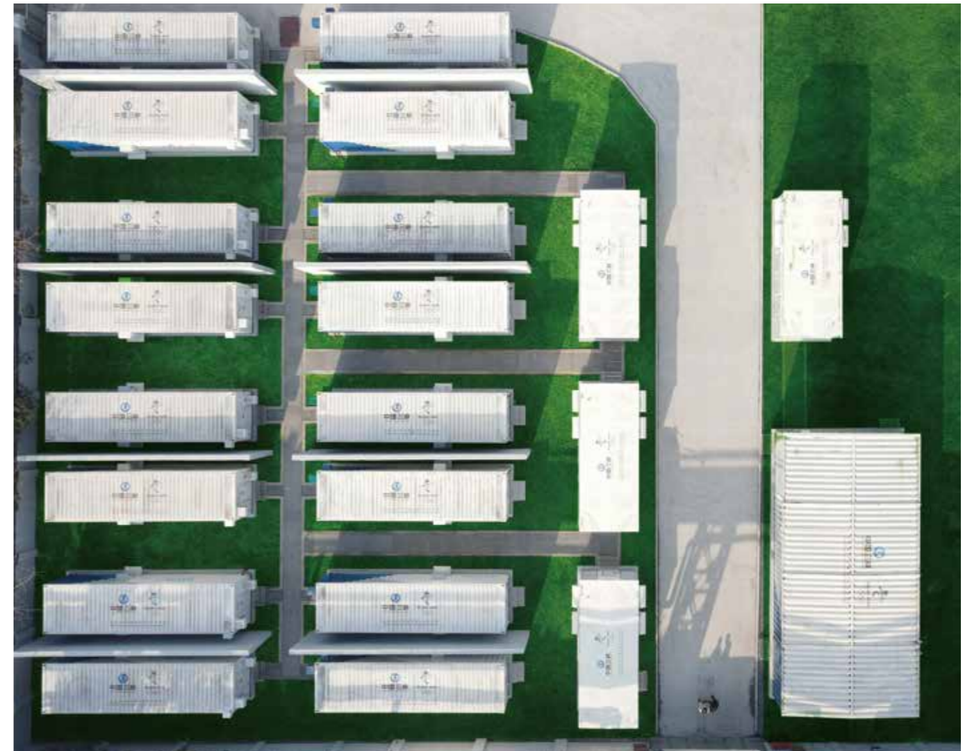
10MW/39MWh Energy Storage Station
