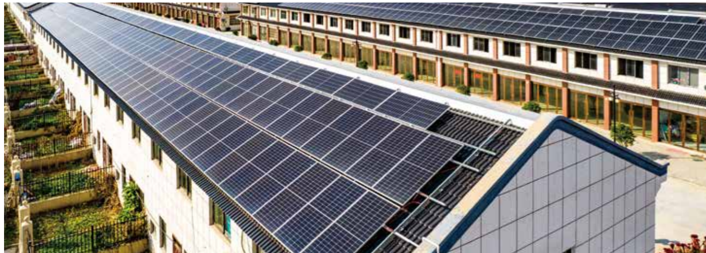
202MW Distributed PV Project (Phase I) of Guannan County, Jiangsu
