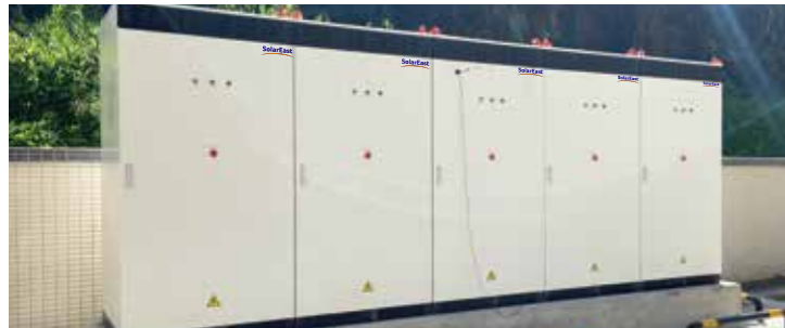
Industrial & Commercial Energy Storage Project, Guangdong
