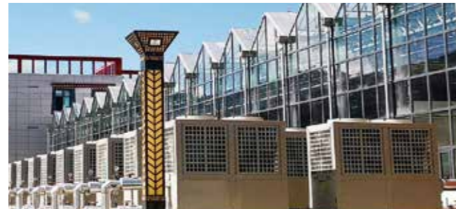
Heat Pump Project, Jingtu Industrial Park in Caina Town, Tibet
