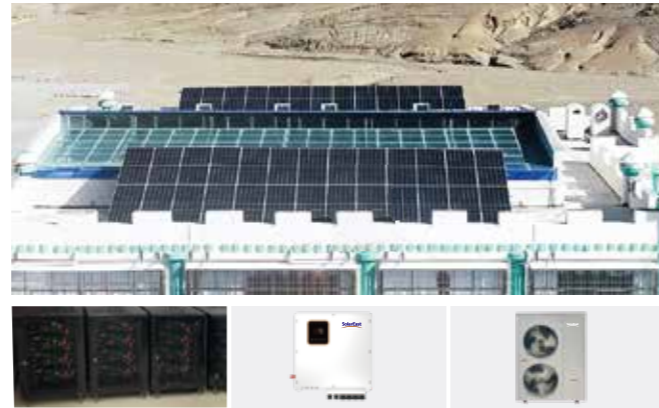
PV+Storage+Thermal project for 17 elementary schools, Tibet
